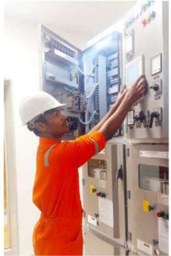
Testing of protection system at Oil Platforms by our protection engineer, Mr. Praveen Kumar
