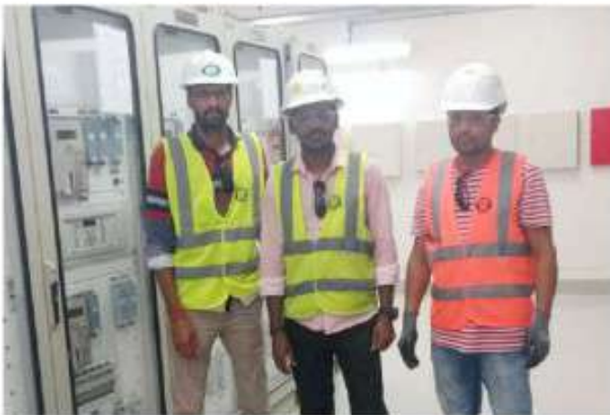
Qatar - 66_11 kV Khore South East Commissioned
