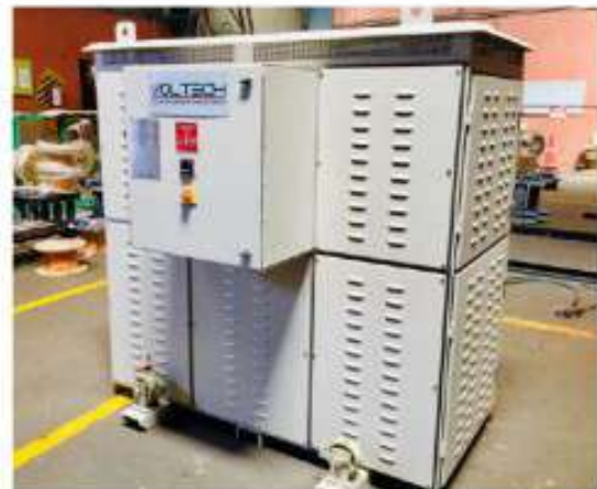
700kVA, 460V/415V, 3-Phase Dry Type Transformer.
